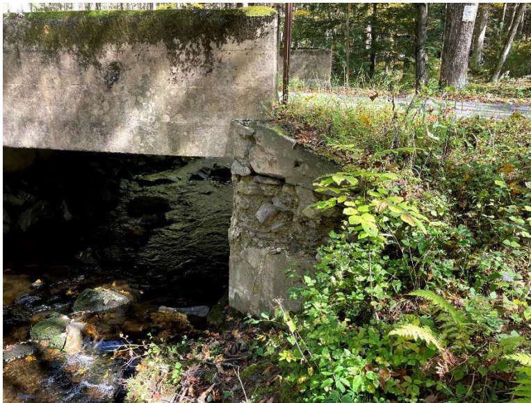
Abutment – Area of Significant Spalling
