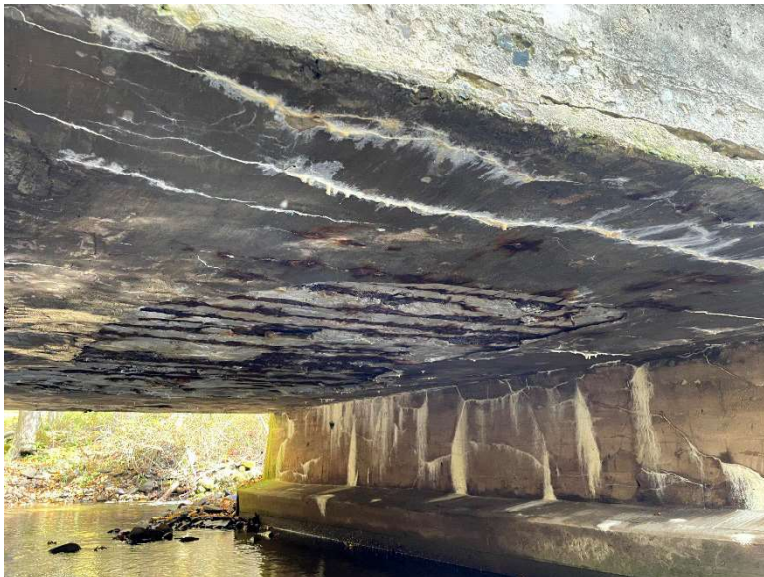
Underside of Deck – Significant Spalling in need of repair
